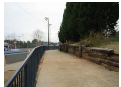
Existing timber wall between Fields Nos. 4 and 5. Wall was replaced with a concrete retaining structure during the course of this study.
